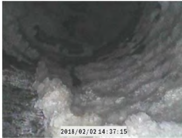
Illustration 125 Typical example of DEF deposits in the CEM mixer assembly
